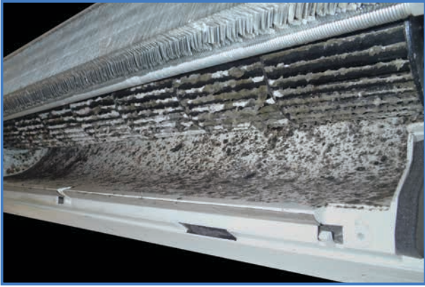
Mini-Split blower with MOLD
